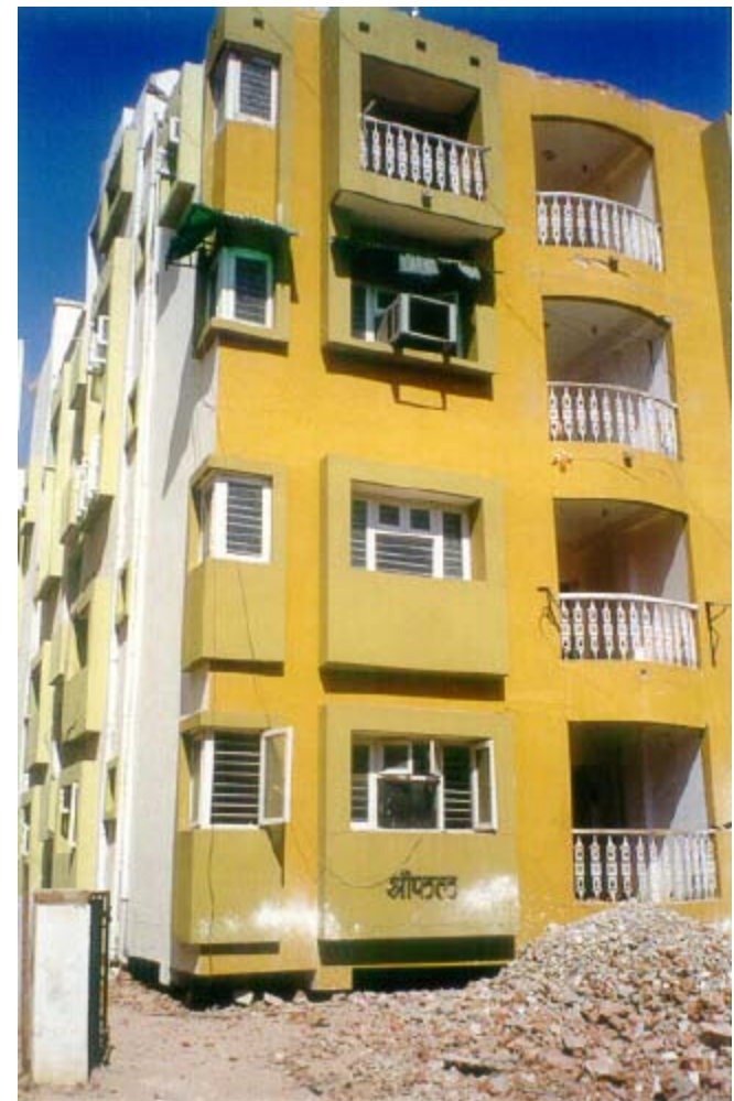
Figure 10-28. Collapse of apartment building in Ahmedabad owing to open ground story failure. No structural damage is observed in the upper stories.
