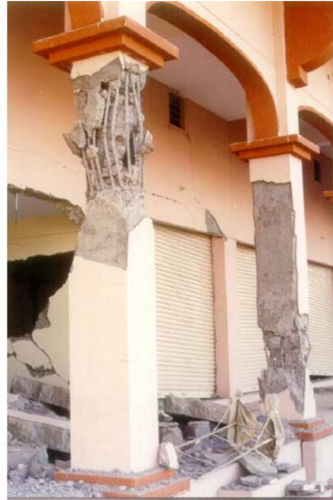
Figure 10-32. Many open ground story buildings did not collapse, but sustained severe damage to the columns in the ground story.
