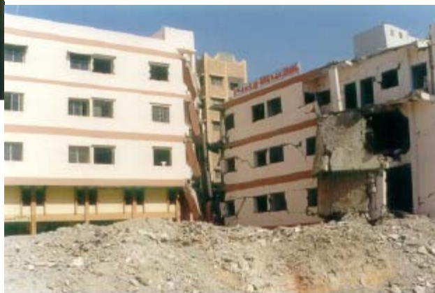
Figure 10-37. Open ground story collapse of short wing of same building.
