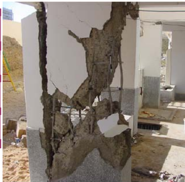
Figure 10-27. Shear cracking of nonductile columns of an open ground story building in Rhu
