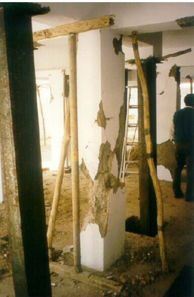
Figure 10-33. Shear failures in columns due to inadequate confinement reinforcement.
