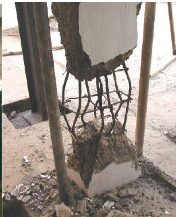
Figure 10-35. Disintegrated concrete within reinforcement cage.
