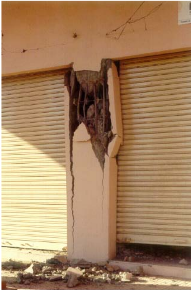
Figure 10-31. RC columns sustained severe damage. Shutters were down at the time of the earthquake.
